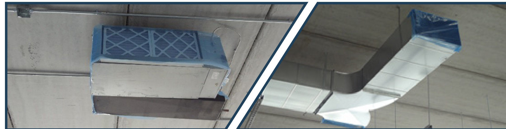
Figure 8: Air Handling Equipment Temporarily Sealed During Construction
